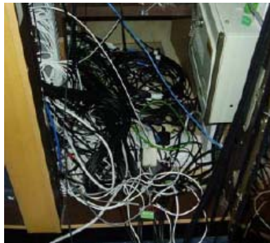
An example of poor quality installation
